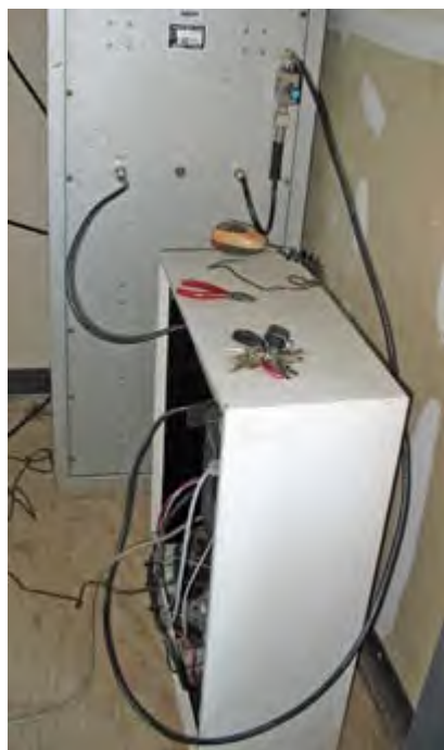
2 meter 'test' repeater installed at Putnam Valley site in 2007. Large cabinet houses a 6-cavity duplexer.
