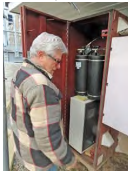
Bob tests the new MTR3000 repeater on February 12, 2024.
