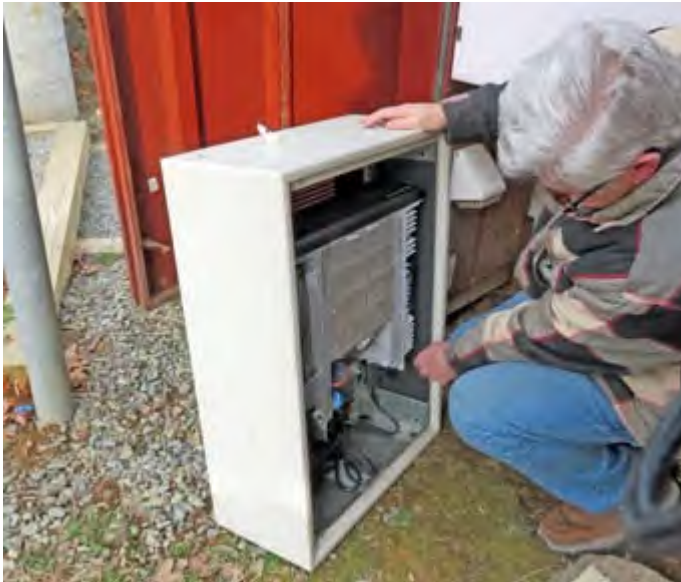
Bob N2CBH prepares the new 2 meter repeater for installation on the hill, February 12, 2024.
