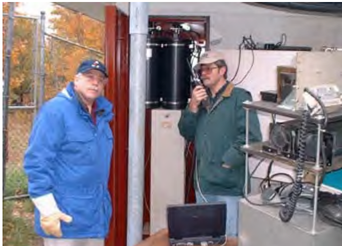
Greg KB2CQE and Bob N2CBH test the new 2 meter repeater after installation on November 2, 2002. The repeater is in the red-brown metal case, with the duplexer at the top. The old repeater can be seen on the open shelving at right. [From PCUD December 2002.]
