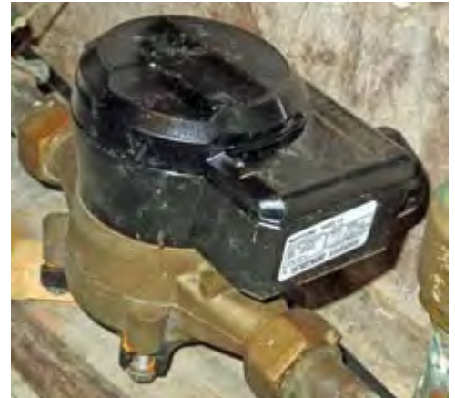
New register head installed on the existing bronze meter body by twisting clockwise and securing with a tamper-proof pin.
