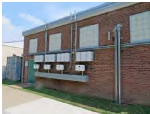
Solar power installation, GW Elementary.
