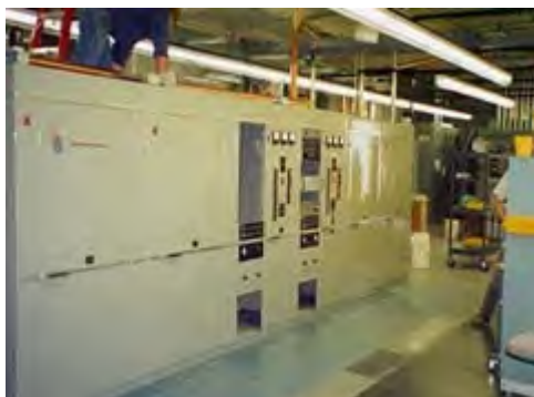
One of the Continental Electronics FRT-72 transmitters installed at WWVB, Fort Collins, Colorado. [Credit: NIST]
