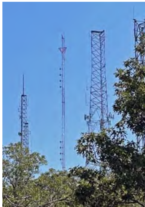
One of four tall towers at the north summit has two 4-bay arrays for WSPK-FM.
